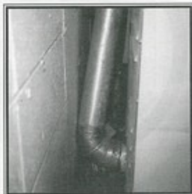
Metal transition duct disconnected at exhaust.
